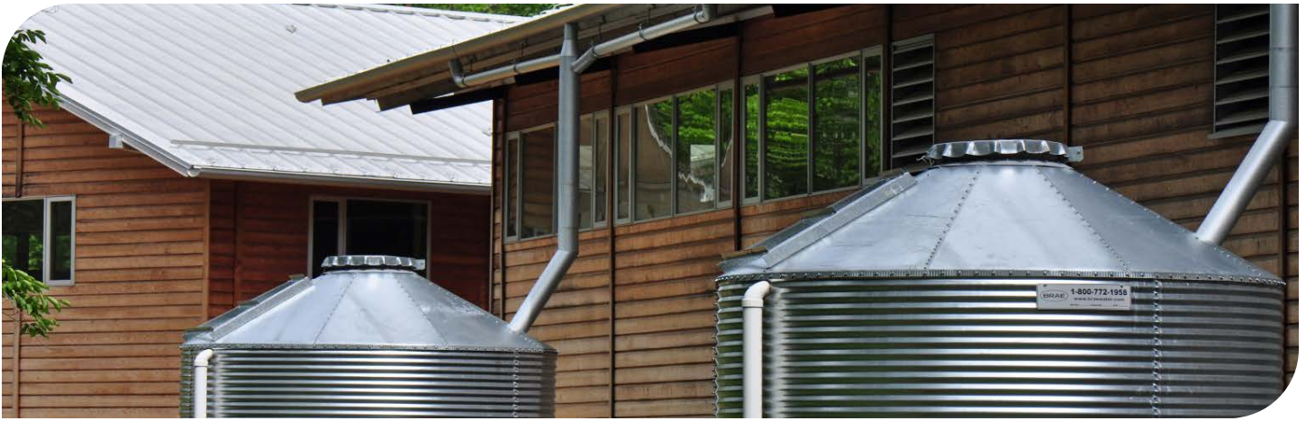
Active rainwater-harvesting systems can be scaled in size and complexity based on water needs.
